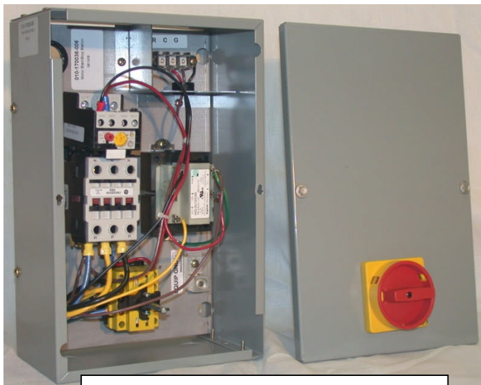
Figure 2 MSS, cover removed – with Starter and Overload
